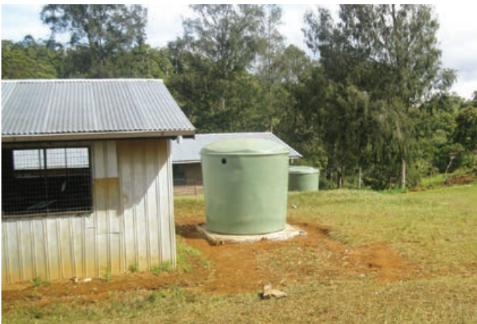
A new water tank installed at Idauwi Primary School as part of infrastructure development support in Hides
