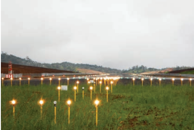
Runway lights at Komo Airfield
