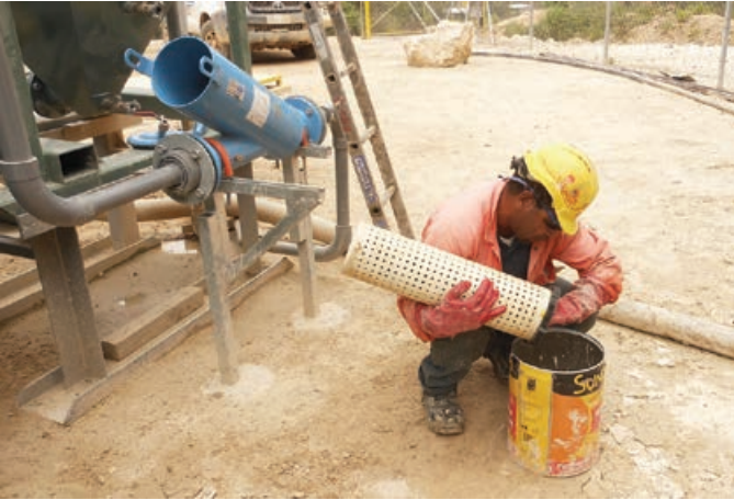
Removal of trapped seeds at the Hides Permanent Vehicle Washdown Facility
