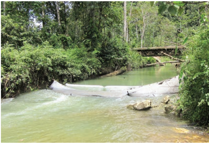
Installation of sediment booms and curtains prior to pipeline installation across the Tugibu River
