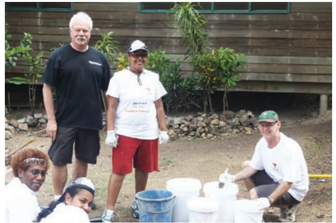
Project volunteers with City Mission workers preparing to re-paint rooms in the Mission
