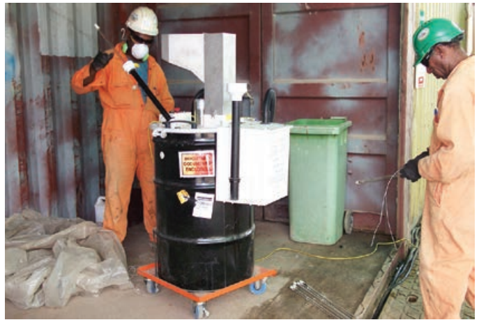
Disposing of ultra-violet lights removed from wastewater treatment plants
