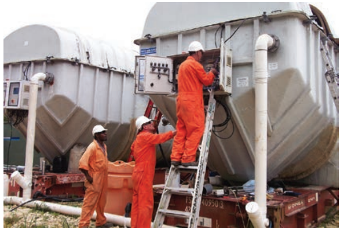
Suppliers performing annual maintenance checks on wastewater treatment plants
