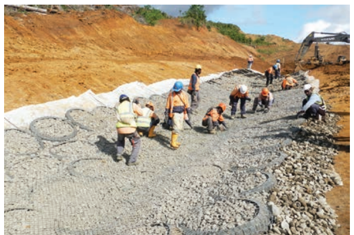
Construction of permanent lined drain at the Komo Airfield using Ecoflex units
