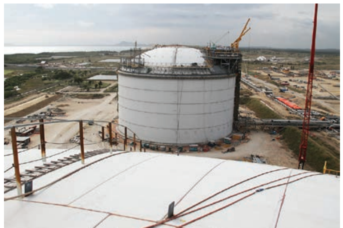
The north LNG tank as seen from the top of the south LNG tank
