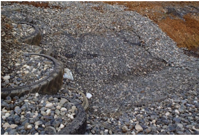
Tires reused as Ecoflex units and then filled with aggregate to provide erosion control structures
