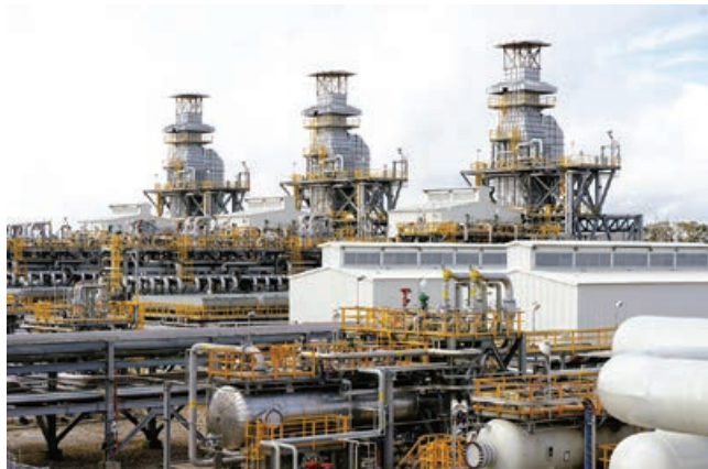
HGCP liquids handling equipment (foreground) and three pipeline compressor exhaust stacks
