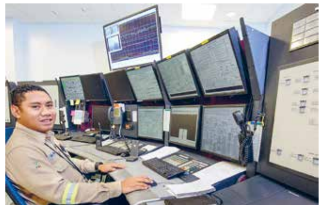
Plate 5.4 – Utilities, Storage and Loading Control Room Technician, Dairy Pota, working in the LNG Plant control room
