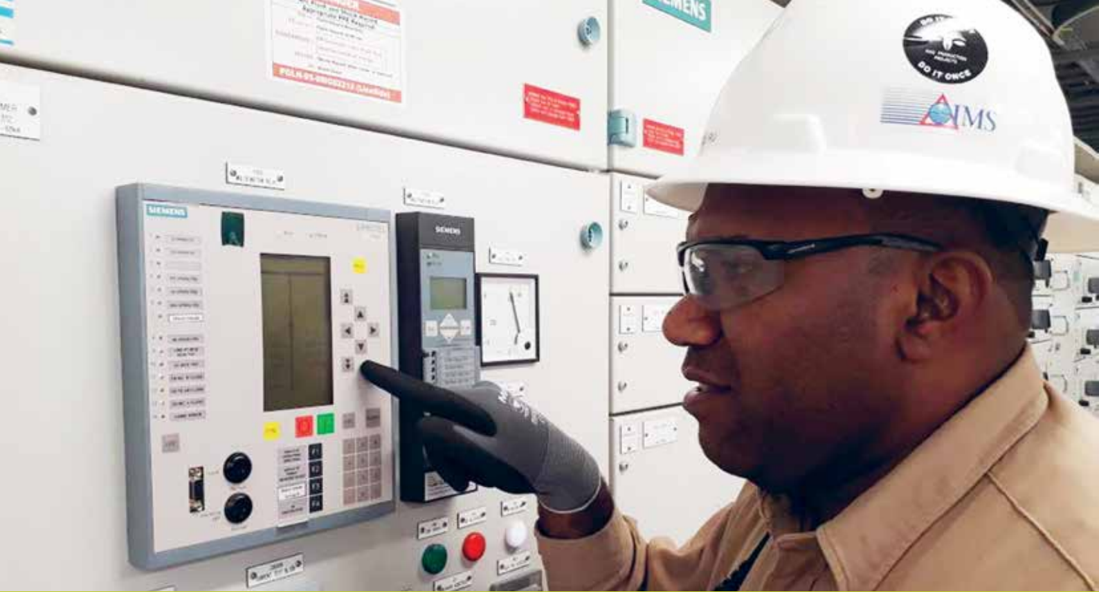
Electrical Engineer, Lei Banduru working on a switchgear protection relay at an LNG Plant substation
