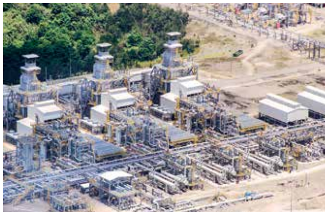
Plate 1.1 – Aerial view of the HGCP gas processing units and pipeline compressor units
